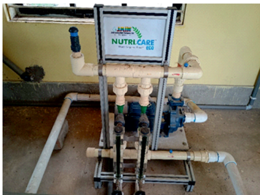
Drip irrigation controlling valves
